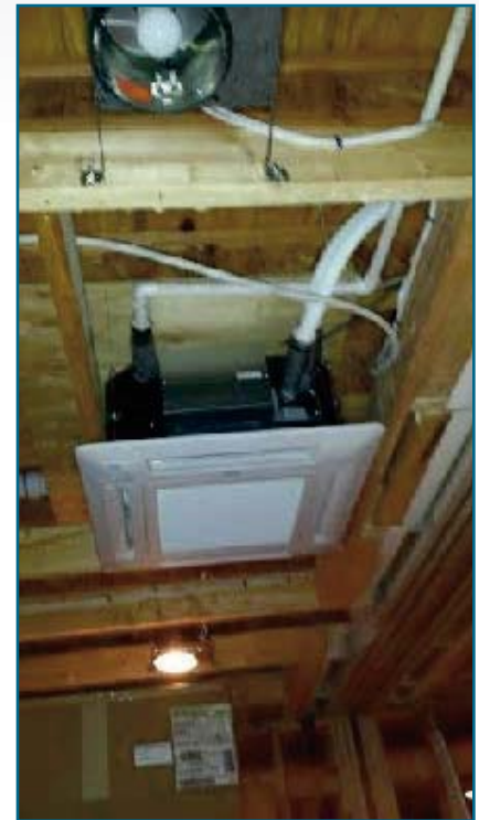
Ceiling cassettes were installed between floors and in the attic. Since the house was gutted, all piping ran neatly inside the walls.
