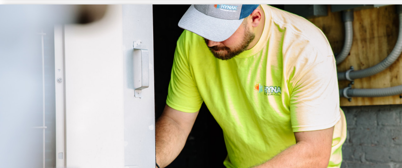
Nick Hynak, partner at Hynak Air Conditioning & Refrigeration, helps commission the VRF systems at The Ritz.
