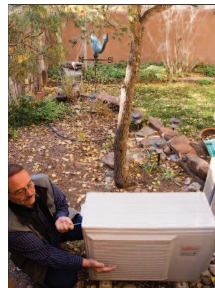
Joe Salazar performing routine maintenance inspection on one of the five one-ton Fujitsu heat pumps installed in a Santa Fe residence
