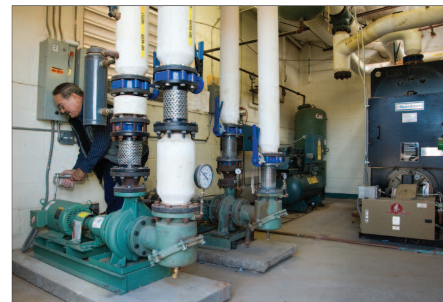
Joe greases Taco recirculating pumps at the K-4 campus of Pojoaque Valley Schools.
