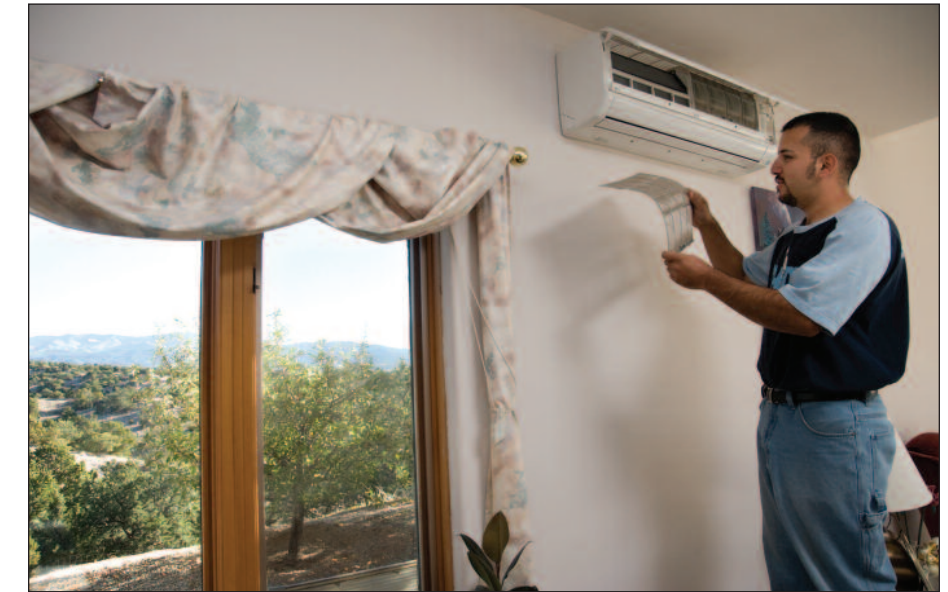
Irvin Marin, service technician, cleaning filters on the indoor Fujitsu pump in Joe Salazar's home
