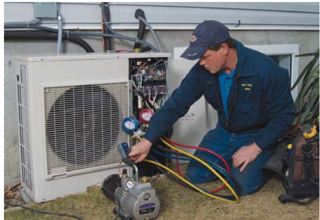
Installation manager Kurt Lehmann checks the operation of the condensing unit. (David Szabo photo)
