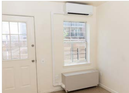
Each unit the Loring Avenue multifamily housing facility is now conditioned with a Fujitsu STHP heat pump system.
