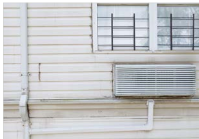
During the retrofit, the STHP outdoor unit is installed within the wall penetration that used to house a PTAC.
