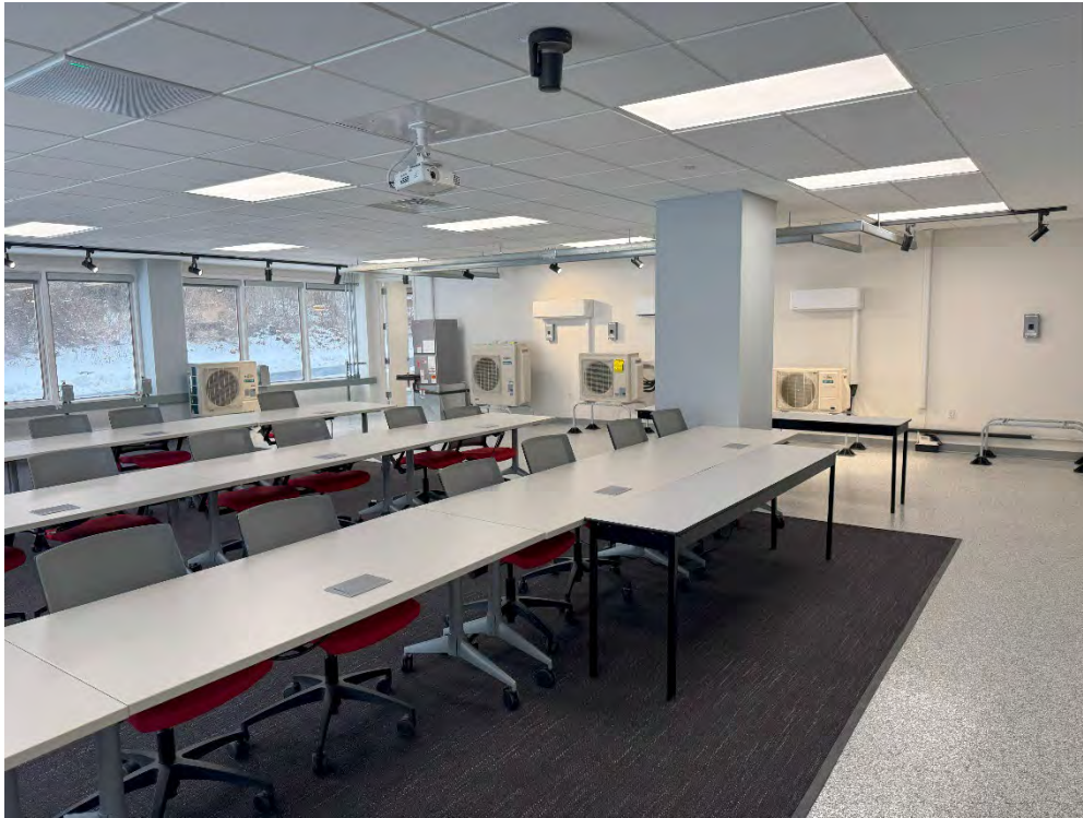
One side of the new training facility features Fujitsu's AIRSTAGE single- and multi-zone residential products.
