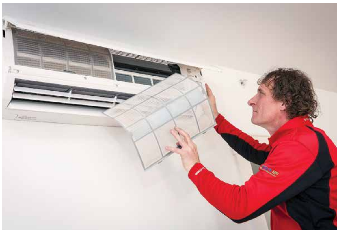
Shearer installs the indoor coil unit on one of 79 Fujitsu RLXFZ units.
