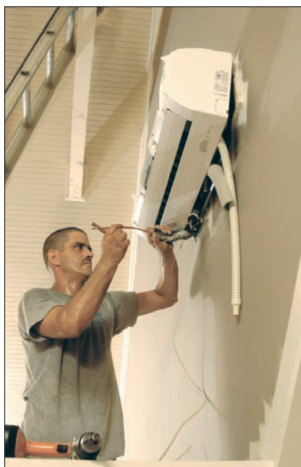
All Pro installer Joel Wasik prepares to connect refrigerant and condensate lines to a Halcyon air handler.
