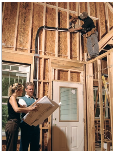
Pam Fasse and employee Tim Lewis, mechanical foreman for the job, review system plans as All Pro installer Joel Wasik prepares refrigerant line sets and the condensate line for one of the home's air handlers.
